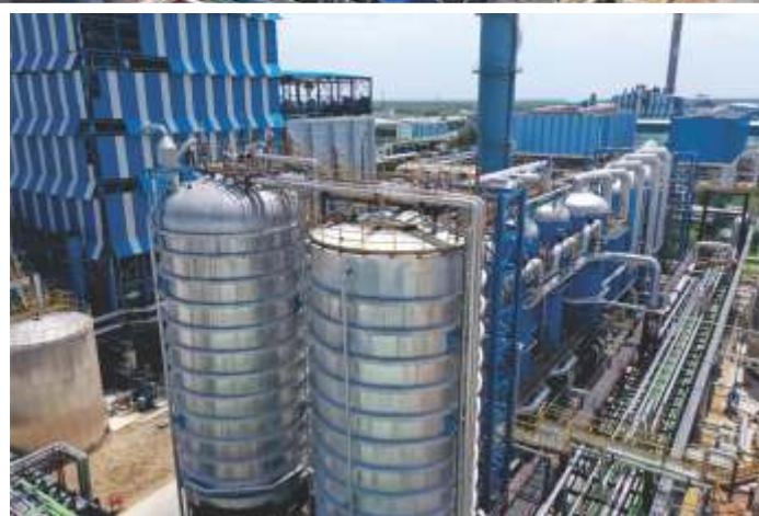
Chemical Recovery Boiler
