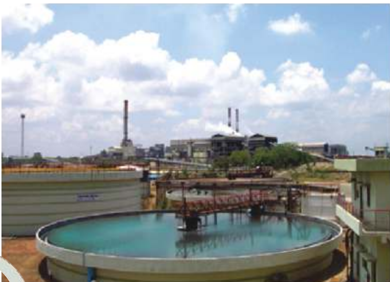
TNPL's modern Bio-methanation plant
