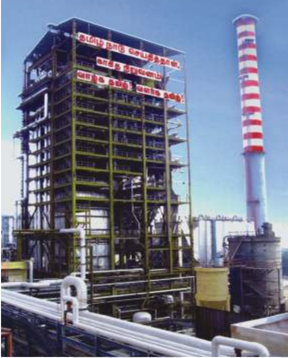
Chemical Recovery Boiler
