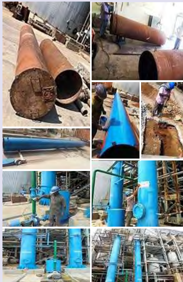
Photograph of stage-wise implementation of the in-house Sulphide stripping column
